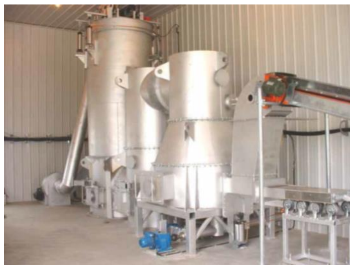
3 MM Btu furnace
